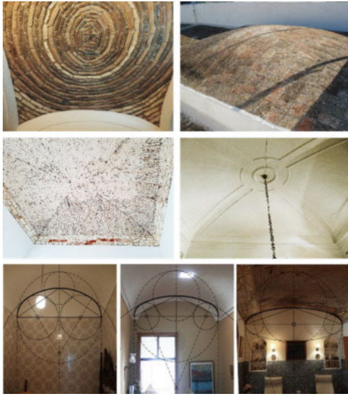
Figure 6. (top) Intrados and extrados of the sail vaults located in the main room casa de fora ; (middle) Intrados of cloister vaults in the main room casa de fora ; (below) Geometrical construction of arch profiles of lowered barrel vaults with three-centred arch, based on in loco measurements (author's photos).
